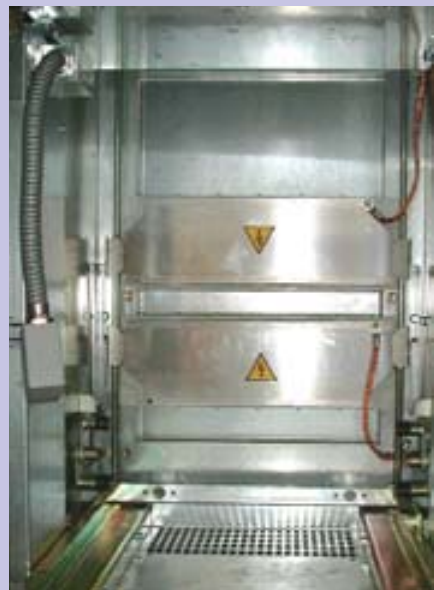
Comparto interruttore Circuit-breaker compartment
